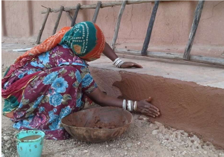
Figure 2.2: Local women of western Rajasthan region performing periodic finishing on mud structure
