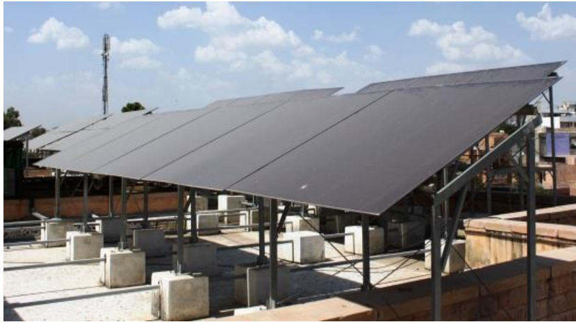
Figure 3.5 A-Si Based 43 kW Rooftop Grid Tied Solar Photo Voltaic System
