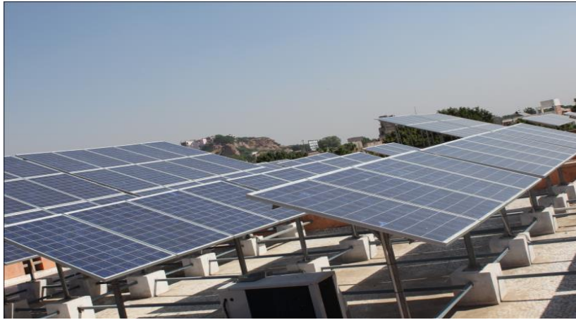
Figure 3.2 C-Si Based 58 kW Rooftop Grid Tied Solar Photovoltaic System
