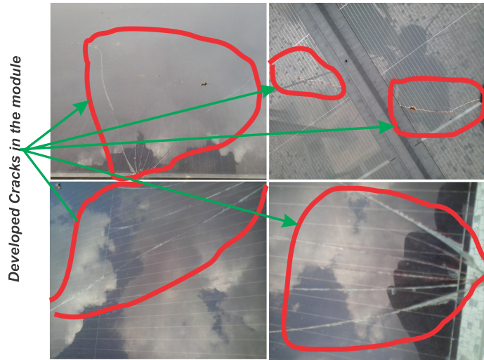
Figure 6.3 : Cracks developed in the PV system modules
